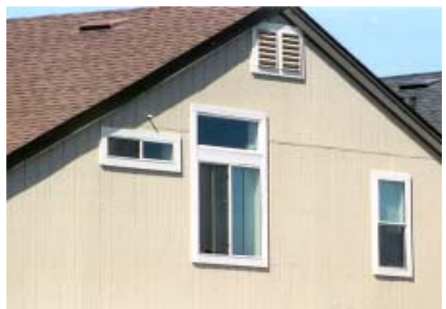
Fig. 3.1.29 These windows are poorly arranged.
