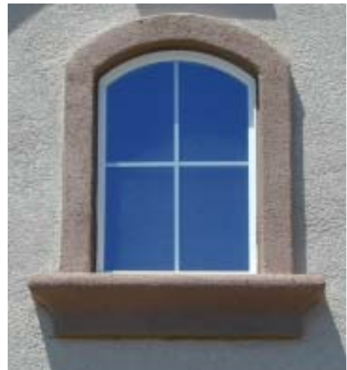
Fig. 3.1.32 Detail, such as this, adds character and interest to homes, and is encouraged.
