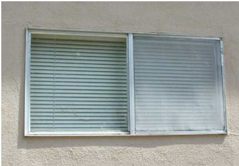
Fig. 3.1.31 Windows set in stucco with no trim or detail are discouraged. This is not superior design.
